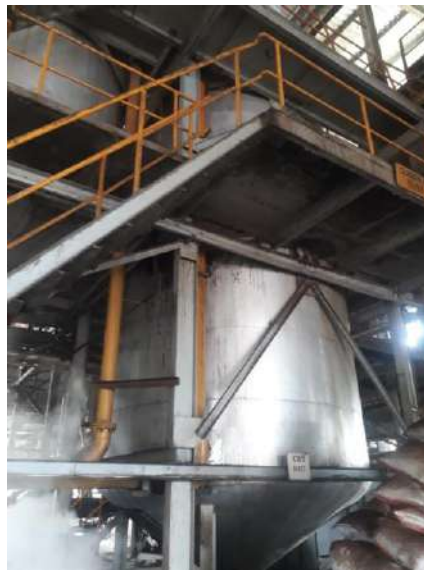
Gambar 1 . CST ( Continuous Settling Tank )
